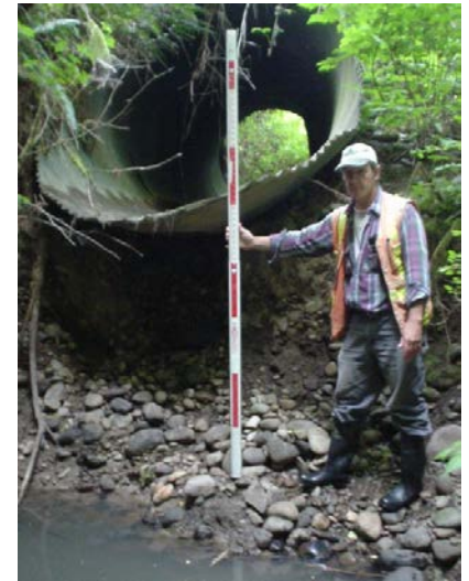
A pipe perched this high above the stream makes it impossible for salmon to migrate upstream.
