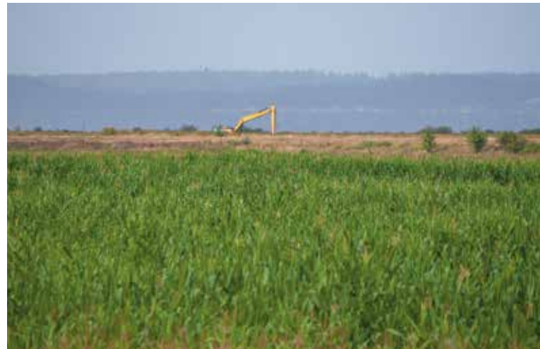
An excavator digs new channels in August, preparing for the Stillaguamish Tribe’s zis a ba II project that will replace corn fields with salmon habitat. Kimberly Cauvel
