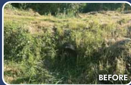
Culverts at Riverfront Park block salmon access in an unnamed creek under a walking trail.
