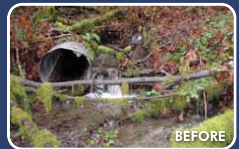
Culvert on Thompson Creek near Rockport creating a passage problem for salmon.
