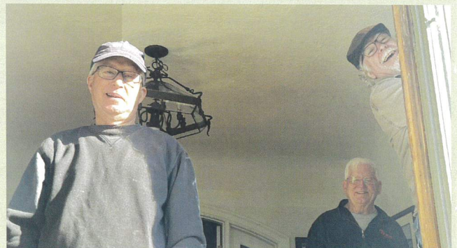
Above: Phil (left), Hal Lee (center), and Paul Engels (right), installing new windows at the SLT office.
