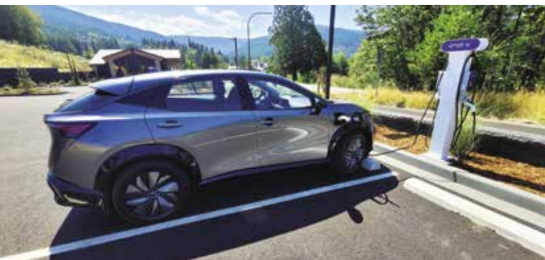
One of the new electric car charging stations installed on the Jamestown S’Klallam government campus. Jamestown S’Klallam Tribe
