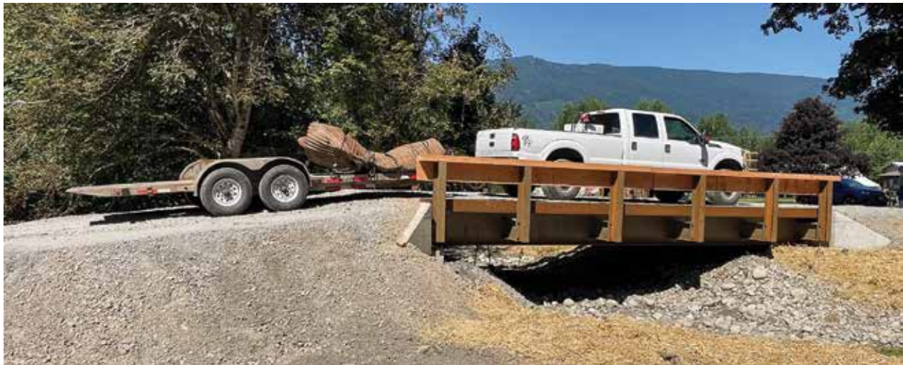
A rusted, undersized culvert removed from Green Creek is taken across the bridge that replaced it in 2024. Skagit River System Cooperative (2)
