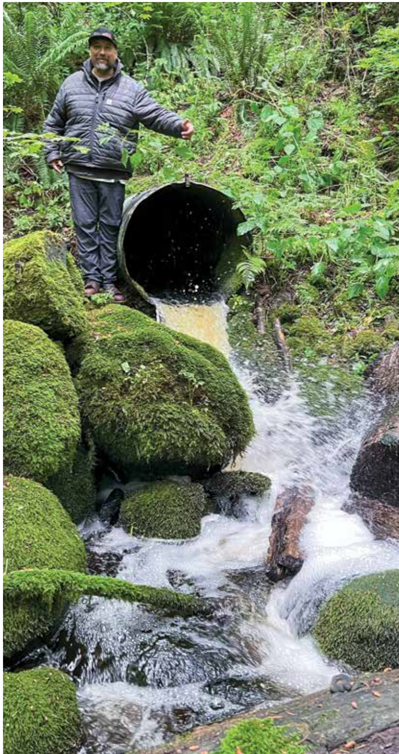
Nisqually natural resources manager James Slape Jr. inspects a culvert on Brighton Creek. The tribe and partners plan to replace the culvert, a project that will open 6 miles of salmon habitat. Nisqually Indian Tribe
